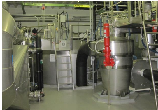
Spray Dryer (Upper part)
