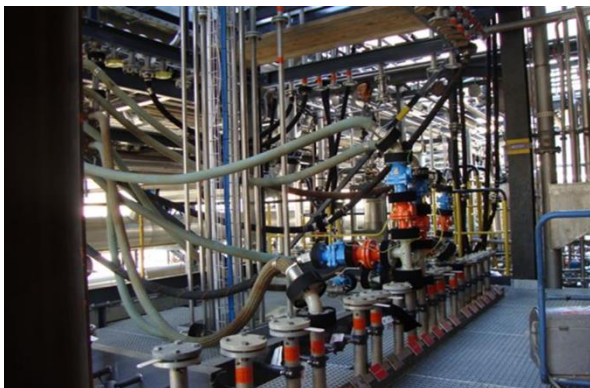
Coupling station for connection to glass line, and stainless steel line
