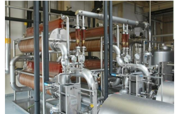
Ultra Filtration Unit
