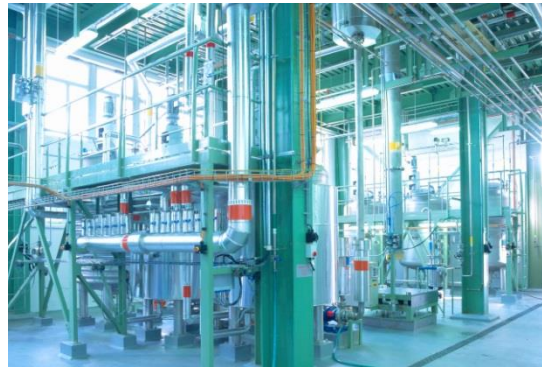
Down Stream Process Plant
